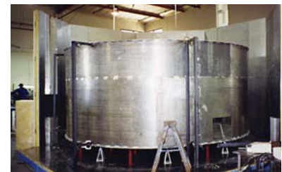
Fluid chiller conditioned stainless steel thermal shroud inside an octagonal prefabricated Bemco chamber under construction.
